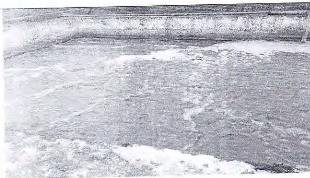
Aeration Tank of ETP
