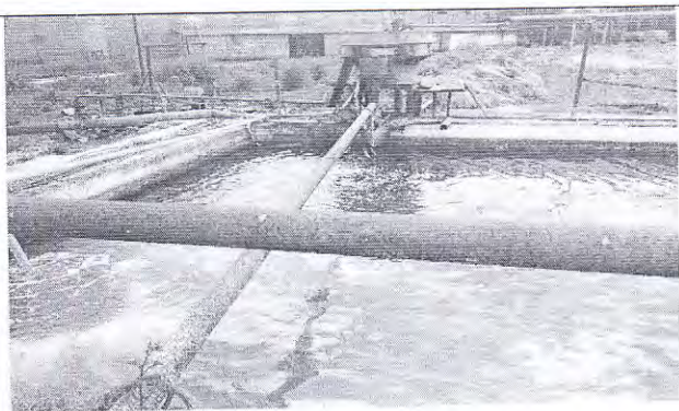
Collection Tank of ETP
